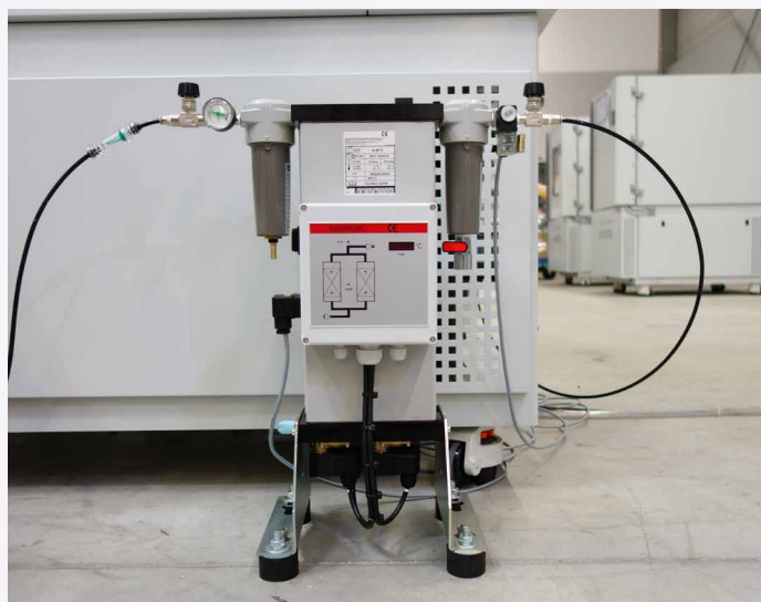
Compressed Air Dryer
